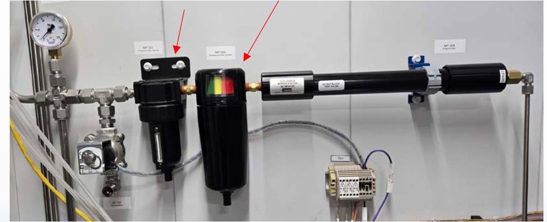
Primary and Secondary Air Filters
